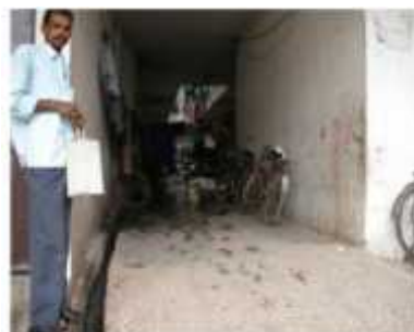
NARROW APPROACH AND INDEQUATE SOURCE OF LIGHT
