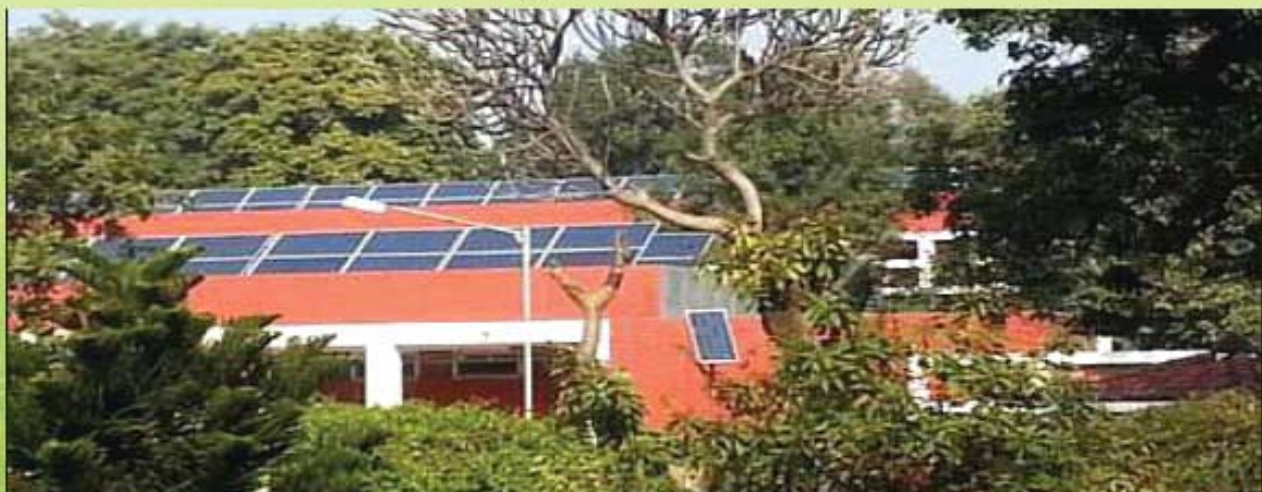
495KWp SPV Power Plant at Govt. College for Girls Sec. 11, Chandigarh.
