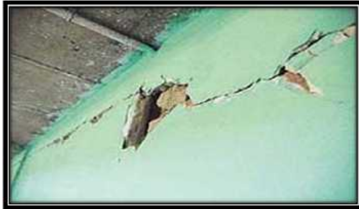
MILD CRACKS ON THE WALLS OF THE SECTOR 42 INDOOR BADMINTON HALL AFTER THE EARTHQUAKE IN CHANDIGARH ON 08-10-2005
